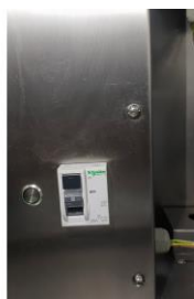
Main power switch and circuit breaker panel
