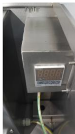
Omron digital temperature controller, mounted inside the cabinet door
